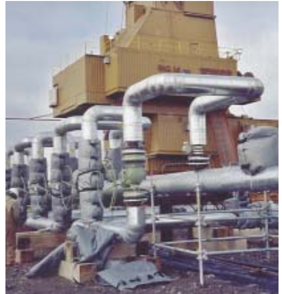
Valve blankets on the S Pad water injection lines. A Doyon drill rig is in the background.
